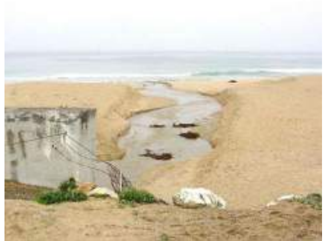
Stormwater Outfall in Seaside.
